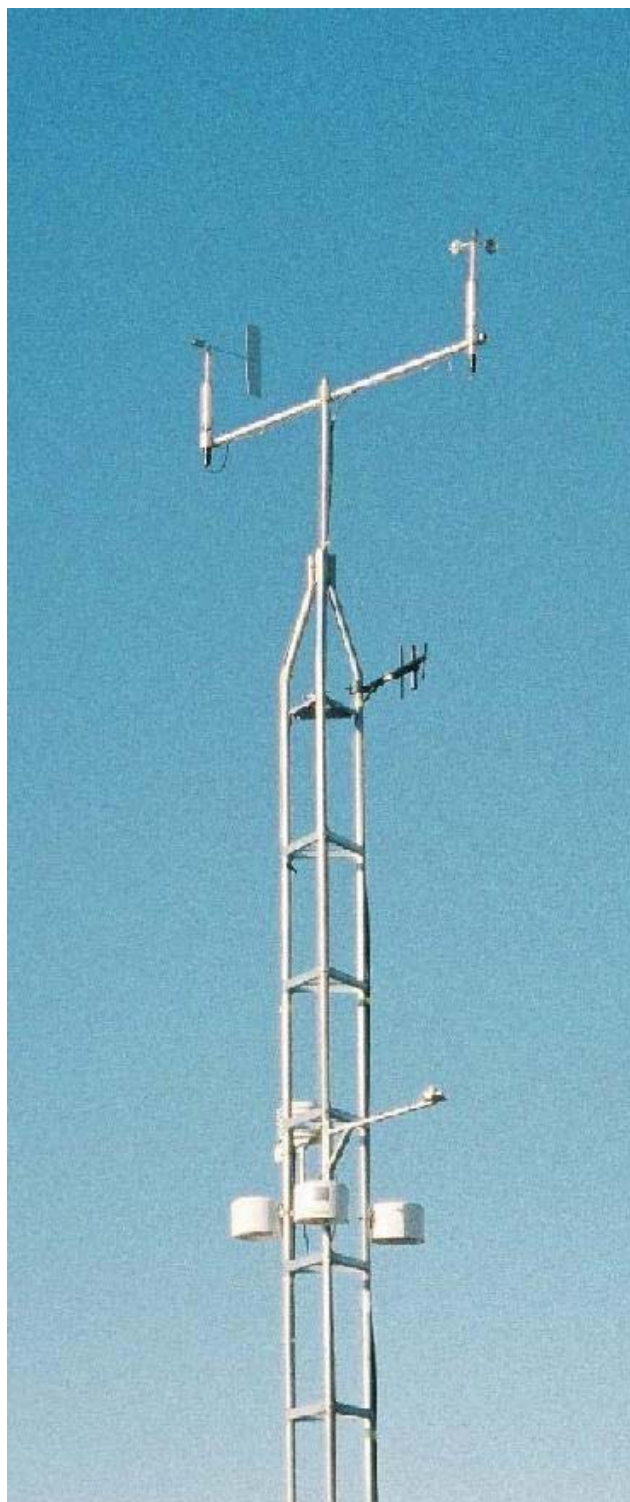
Meteorological Tower and Sensors for the Portable Continuous Monitoring Station
